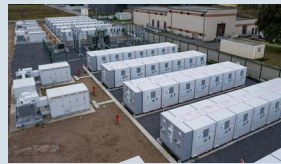
Ruien Power Plant
